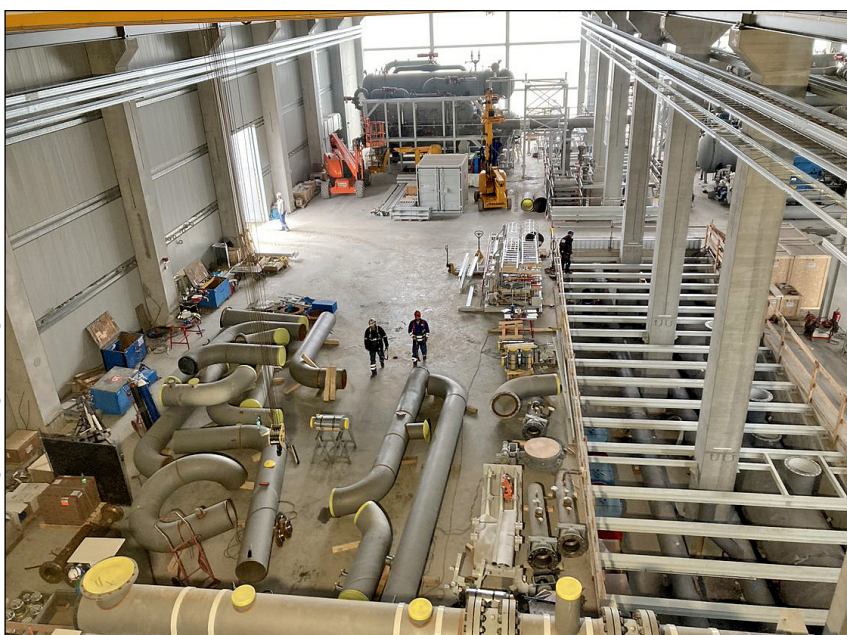
At the beginning of 2023 Wien Energie started installing the first three out of six planned heat pumps
