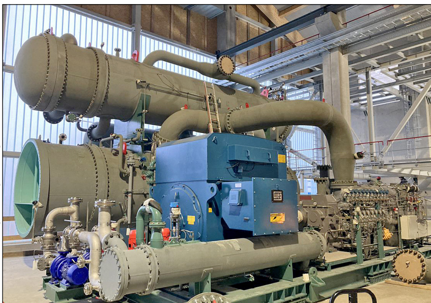
One of the three heat pumps next to the waste-water treatment plant that is now already producing climate neutral heat for Vienna's households
